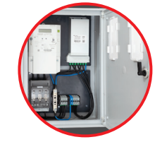
PLC meter and PLC filter in meter box
